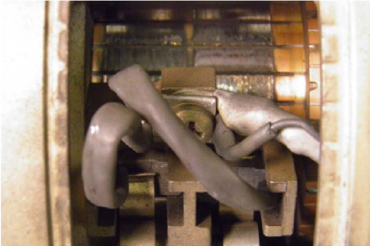
Figure 3.5: Commutator Unserviceable Condition Example
